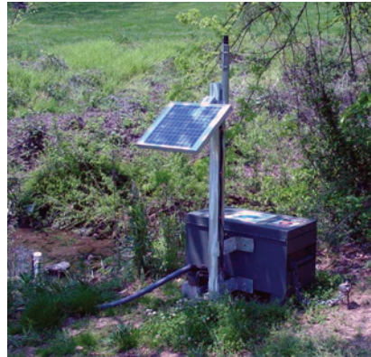
CMANN deployment site with YSI 6820 and solar panel.
